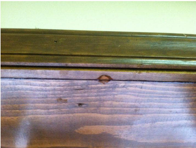
Leakage at the Moncure location in the entrance
