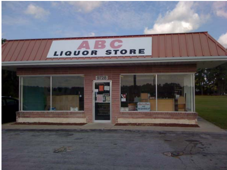
Holes in parking area. Parking area does not have definitive parking spaces.
